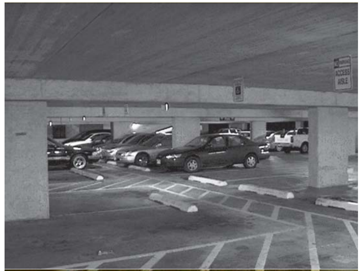
Pictured below: Garages with HID-type (high-density discharge lighting) can save a remarkable 70% on energy usage and 50% on maintenance costs by converting existing fixtures to more efficient RGB fluorescent lighting systems.
